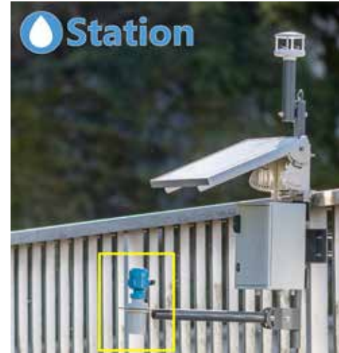
Ogoxe hydrological station installed at a bridge © OgoXe
